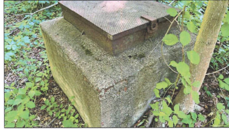
71. Looking west at a manhole for a water cistern located along the northwestern property boundary just east of the house in the Shiverick – Fairmount West Protected Property.
