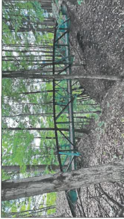
18. Looking north at a metal footbridge that extends over a steep ravine along the northern bluff. The bridge provides a shortcut across the ravine on the northwestern access trail.
