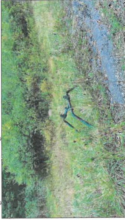
6. Looking north-northeast at gas line apparatus located on the north side of the main access drive in the southeastern portion of the Protected Property.
